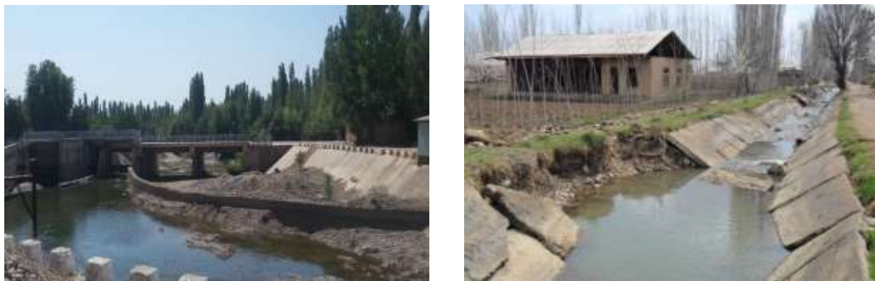
Figure 1. Condition of Govasay hydrosystem station and Left bank canal
