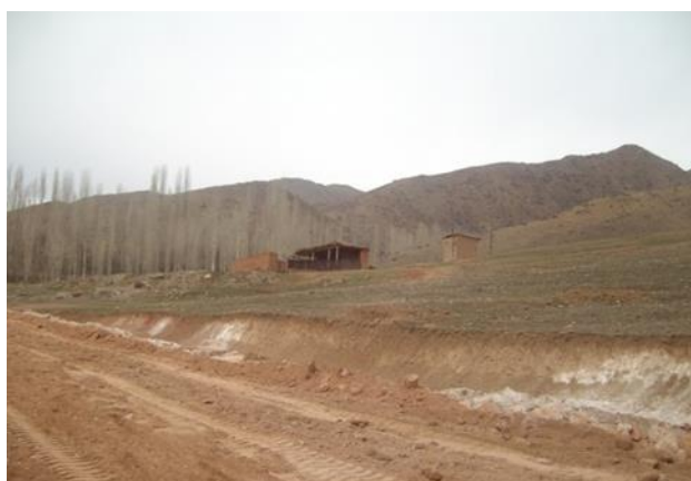
Figure 2. Reconstruction of the highway 4P57 - Kizilkum bypass road: Karmana - Nurota - Boymurod - Utamurod - Mullali - Tomdibulok on the section 22-32 km
