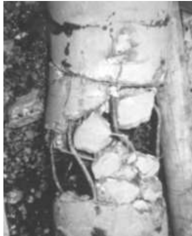
Figure 3. Damage to a pile by 2 m of ground displacement in Niigata earthquake, 1964.
